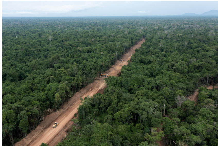
Excavators and bulldozers work on a recently built road cleared through a section of the feasibility study area of KP Cement's mine. Image by Andy Ball for Mongabay.
